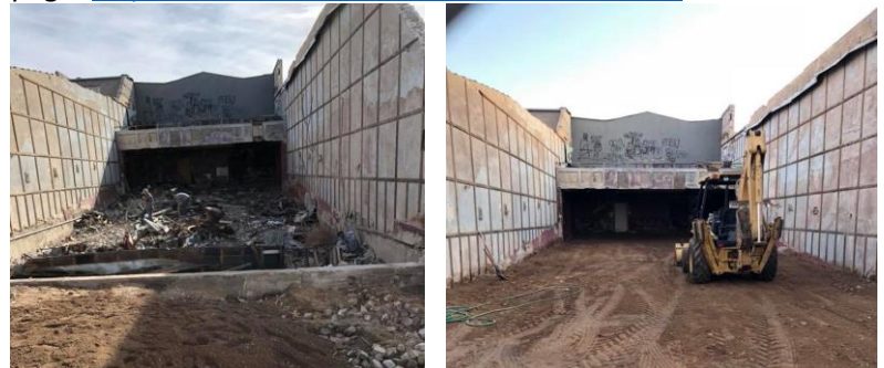
Left: Photo taken during removal of xx tons of trash and debris Right: After removal and ground leveling
